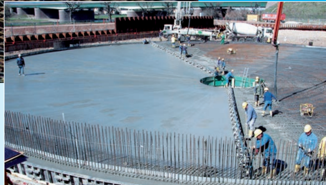
Circular WWTP basin with two large NOGGERATH Variants® - 2.2 operating simultaneously
